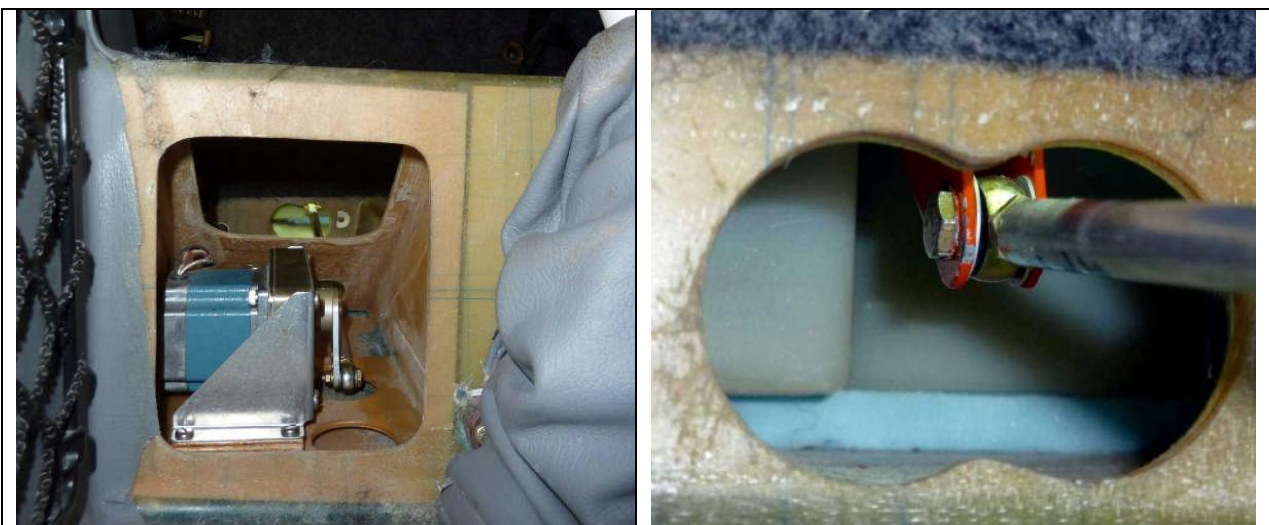
Picture 2 Example TruTrak installation.
